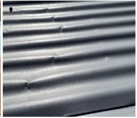
Roofing iron is dented
