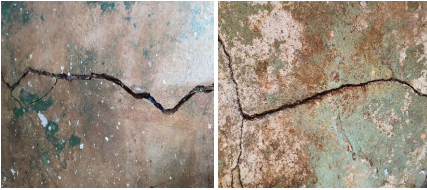
Significant cracking to section of detached building floor
