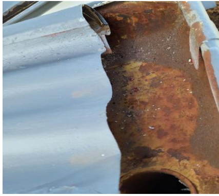
Rust to gutters
