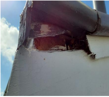
Section of timber barge is missing
