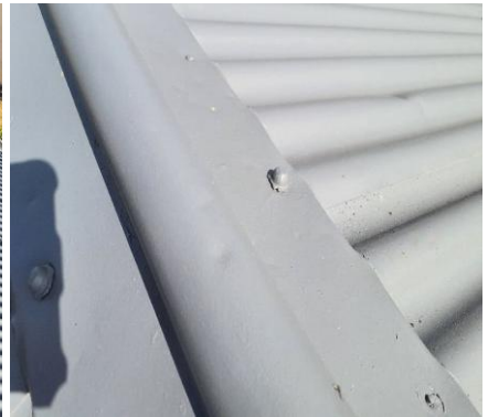
Hail damage to roof exterior
