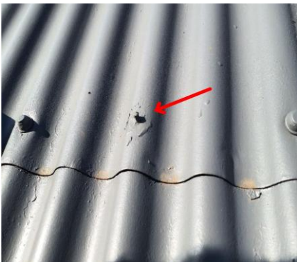
Heads of roofing nails missing
