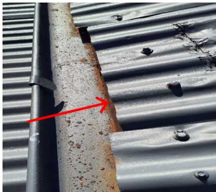
Roofing iron is short
