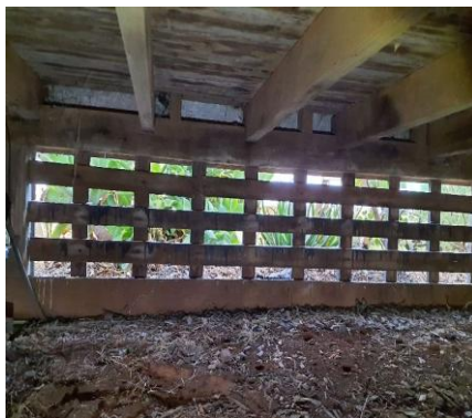
Timber slats in contact with the ground and floor framing
