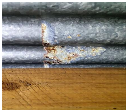
Rust to laps of roofing iron
