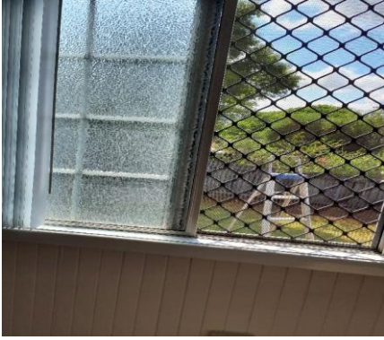
Windows require service
