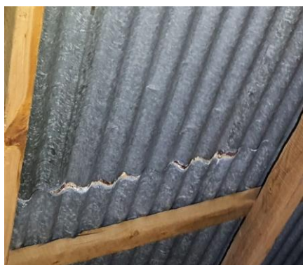
Rust / corrosion to laps of roofing iron
