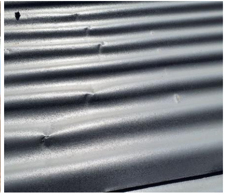
Roofing iron is dented
