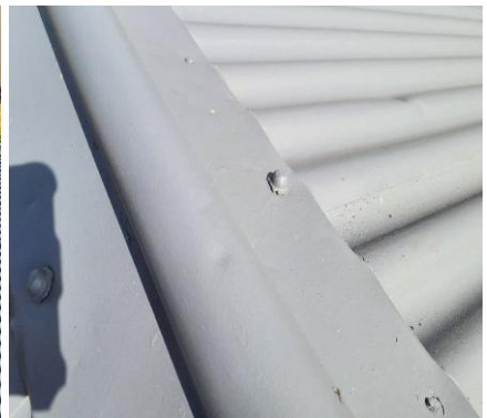
Hail damage to roof exterior
