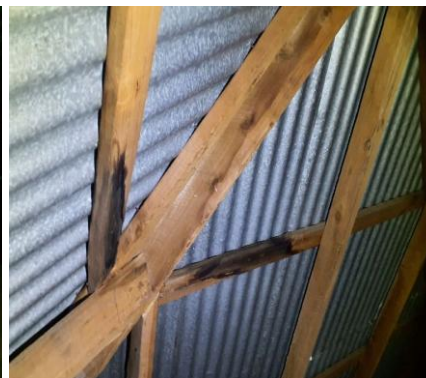
Water staining to roof framing
