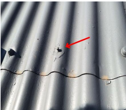
Heads of roofing nails missing
