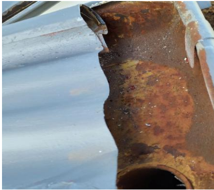
Rust to gutters
