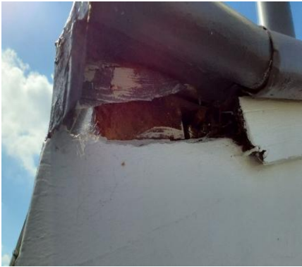
Section of timber barge is missing
