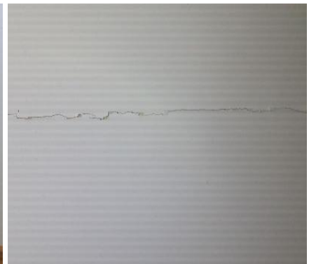
Cracking to the join of the garage ceiling lining
