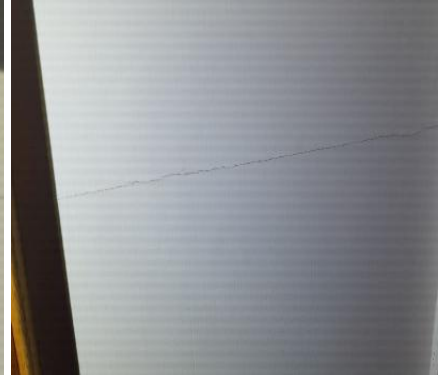
Minor cracking to the join of the bathroom wall sheeting
