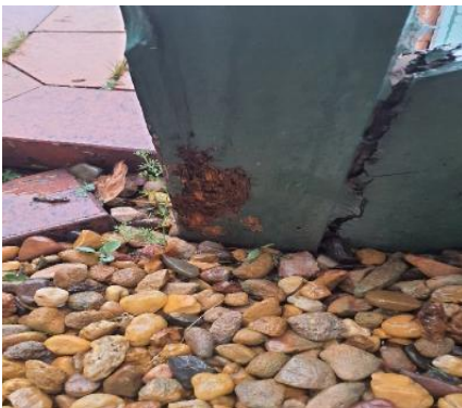
Wood decay to balustrade
