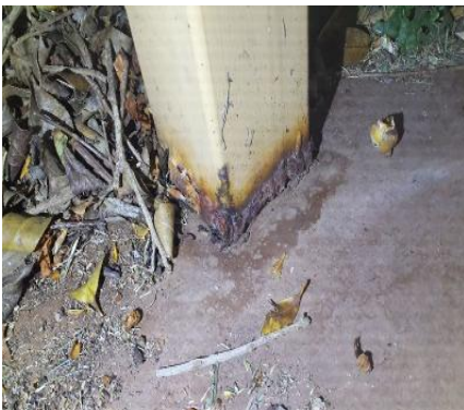
Rust to carport posts
