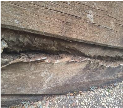
Wood decay to retaining wall timbers
