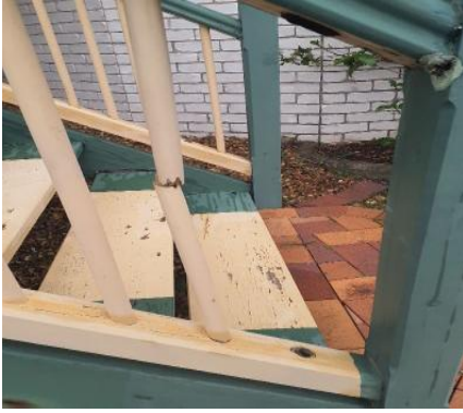
Wood decay, balustrade broken and missing
