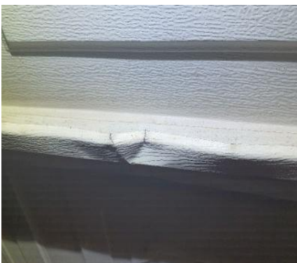
Damage to section of the panel lift door
