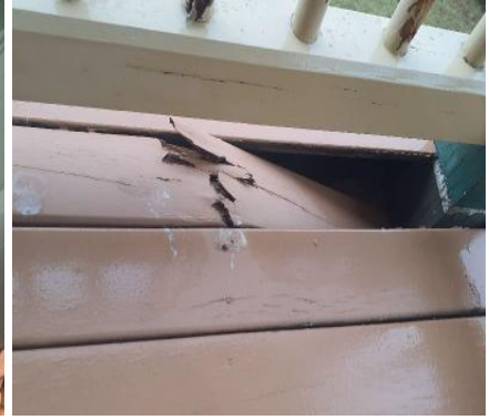
Damage to verandah decking boards
