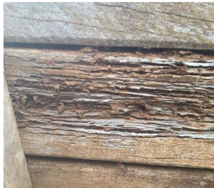
Termite damage to retaining wall timbers
