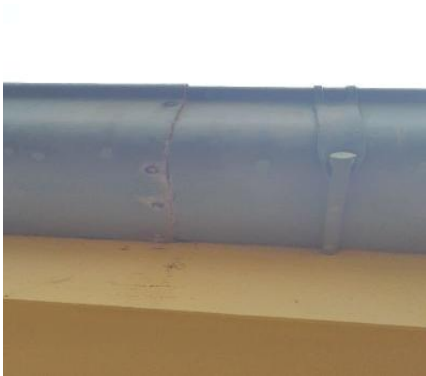
Gutter is leaking on join
