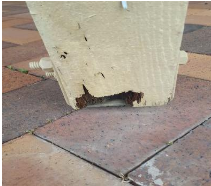
Wood decay to patio post
