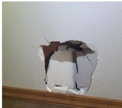
Damage to garage wall lining
