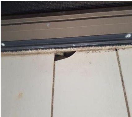
Damaged door sill tile
