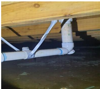
Ensuite waste pipe is leaking
