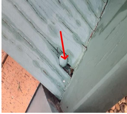
Wood decay to stairs
