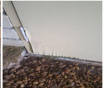
Door to subfloor area has delaminated
