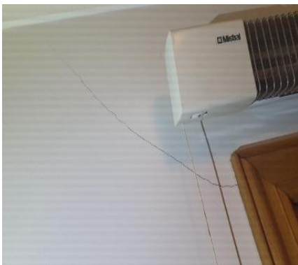
Minor cracking to the bathroom wall sheeting
