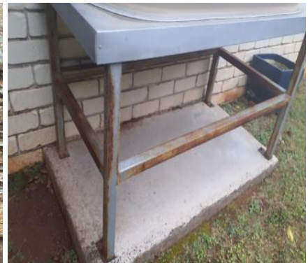
Rust to tank stand
