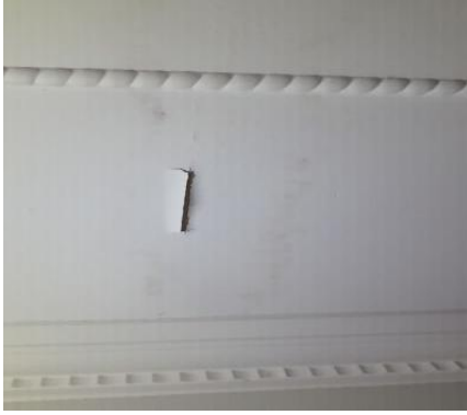
Water staining and paint flaking from section of the lounge room ceiling
