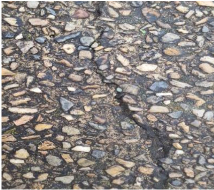
Cracking to the driveway
