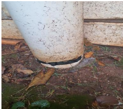
Bottom of the rear downpipe is broken
