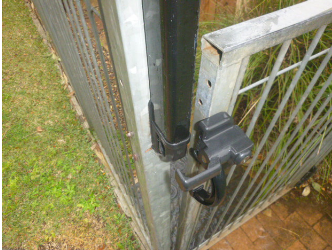
Example showing gate not self-close close to latch
