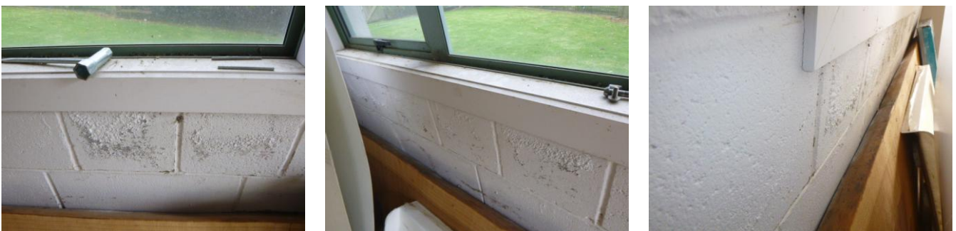
Efflorescence was evident below the basement garage window as seen in these examples
