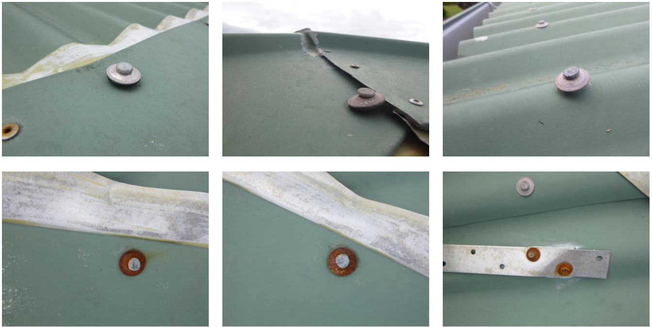
Some loose and corroded fixing were noted on the day of our inspection as seen in these examples
