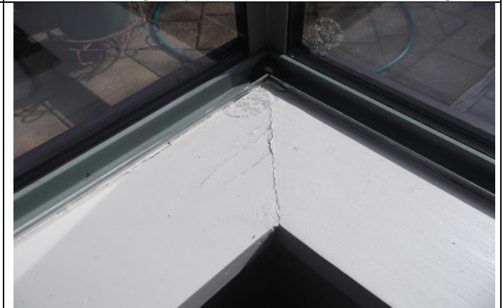
Minor painting required on some window sills
