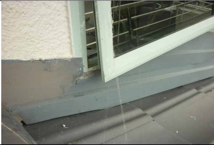
Unusual flashing on upstairs bathroom window
