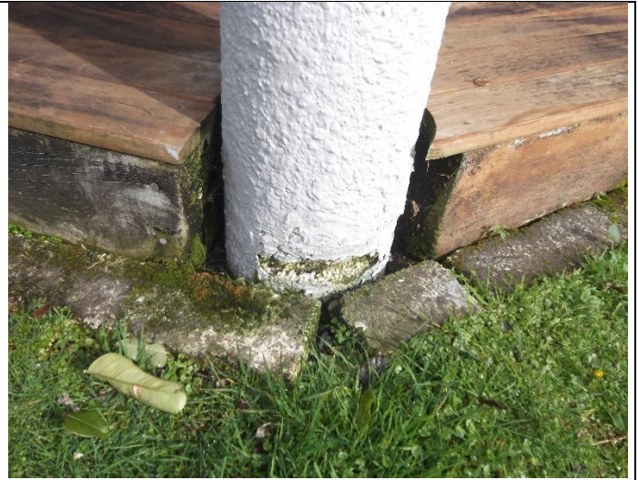
Damage to base of poles possibly by weed eater. Plaster repair required
