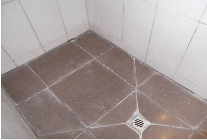
Grout needing repair and silica residue on tiles and grout
