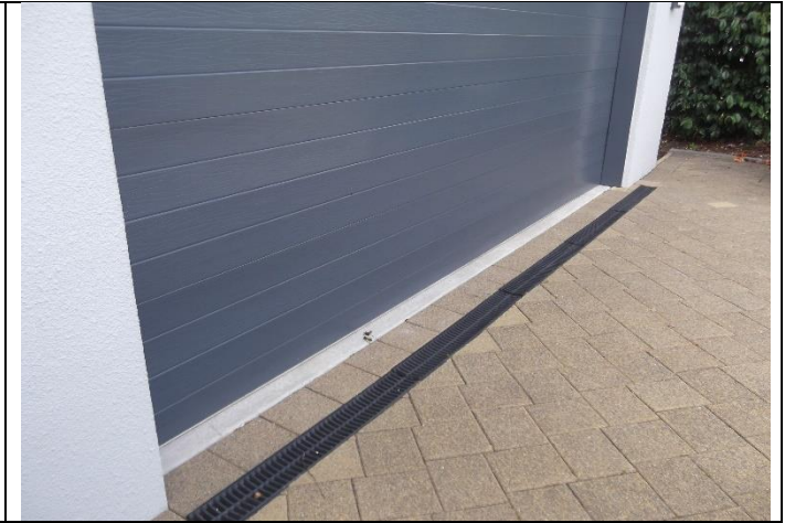
Good collection drain on garage door entrance
