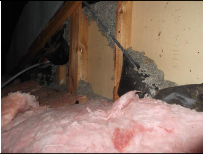
Insulation dropped out of wall above the laundry. This is the upstairs shower wall.
