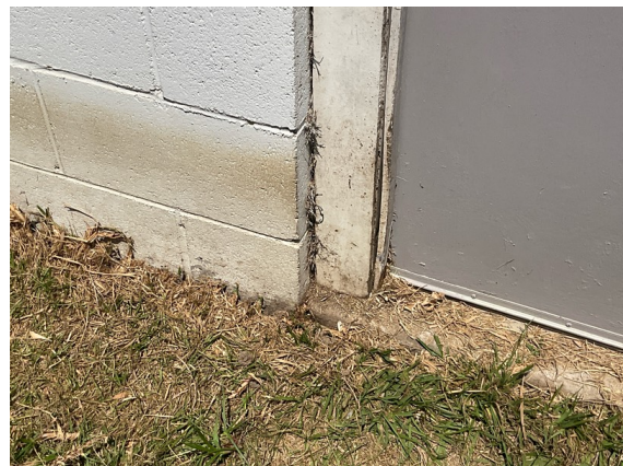
Timber in contact with the ground around the exterior of the home, recommend all timber be a minimum 75mm off the ground.
