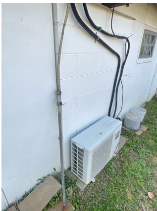
A/C runoff not to a drain, recommend repairs.
