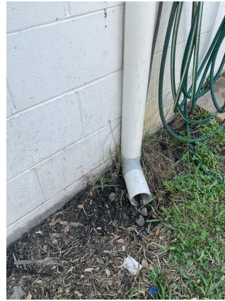
2 x Downpipe's not to drain on the right hand side of the home, recommend repairs.
