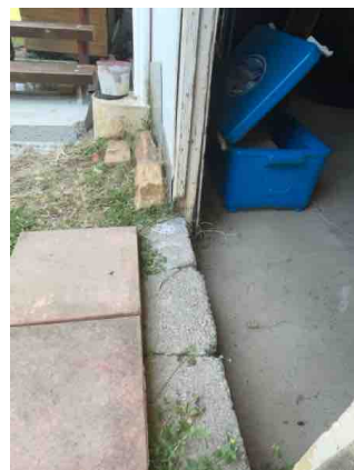
The external ground level is higher than the internal slab along the rear of the building which has lead to moisture issues. Recommend keeping the ground lower than the downstairs slab
