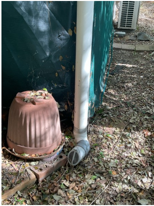
Downpipe on the back patio isn't to a drain, recommend repairs.
