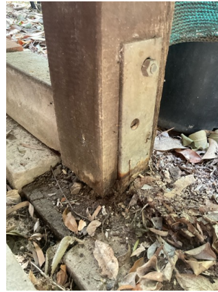
Timber posts on the rear patio are in contact with the ground. Recommend having a minimum 75mm clearance between timber and ground.
