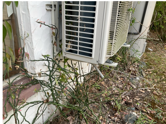
A/C runoff not to drain on the right hand side of the home, recommend repairs.
