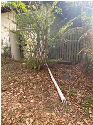
Downpipe not to drain on the right hand side of the home, recommend repairs.
