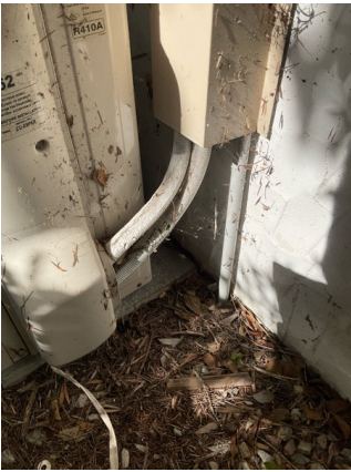
A/C runoff not to drain on the left hand side of the home, recommend repairs.
