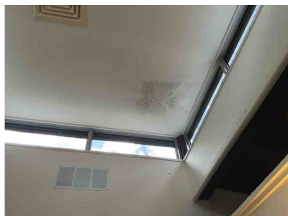
Mould found on the ceiling, recommend repairs.
