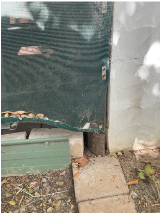
Timber post on the rear patio is in contact with the ground & house, recommend the be a minimum 75mm clearance between the timber & ground.
