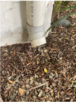
Downpipe not to drain on the left hand side of the home, recommend repairs.
