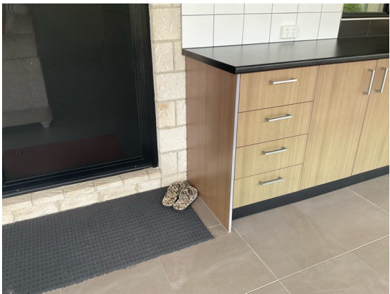
Outdoor kitchen conceals the physical termite management system in the rear patio. Recommend consulting the installers for information on what system they have installed in this area.
